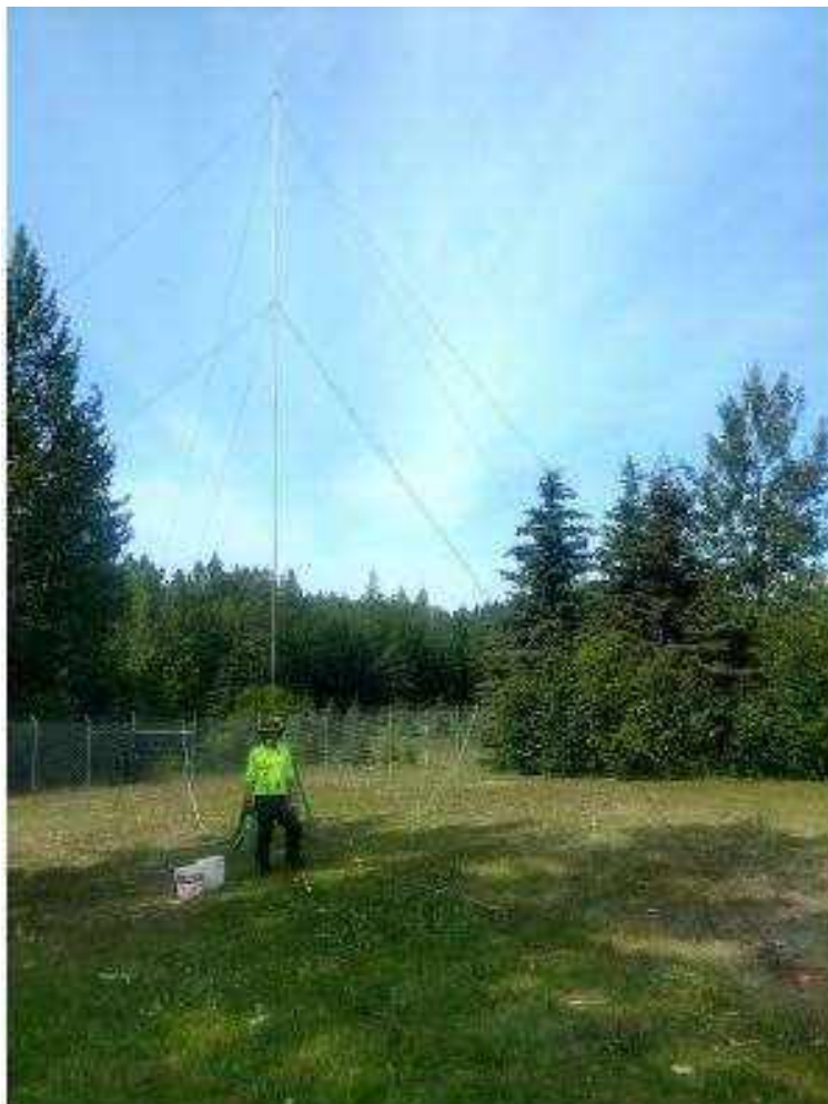
Here is another picture of TJ next to the assembled antenna
