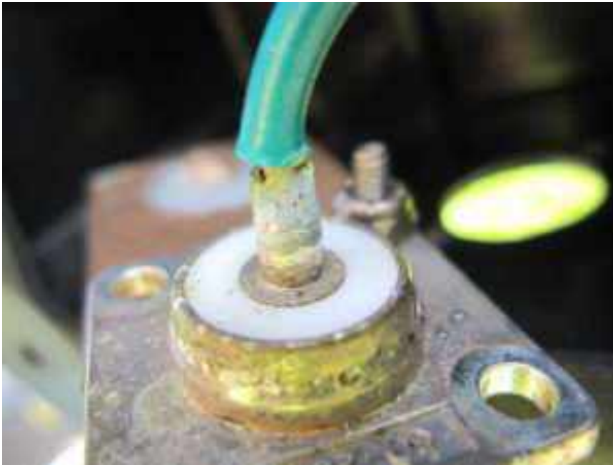
Copper crumbs on the SO-239
